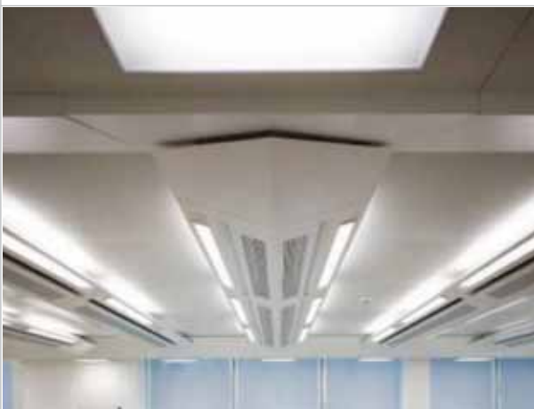
55 Baker St: chilled beam technology
